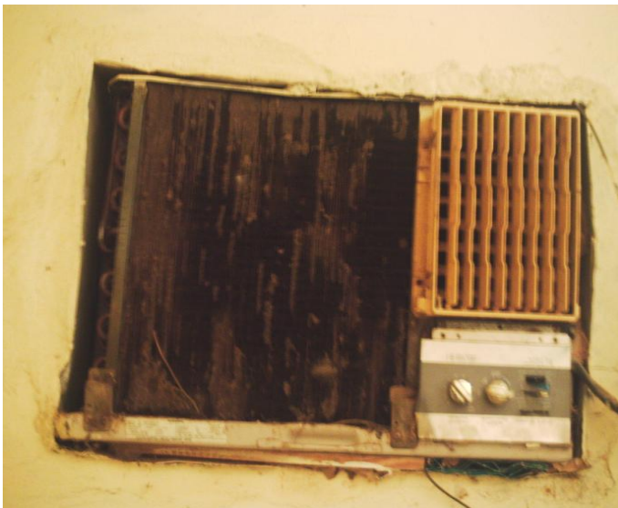
Fig. 1. Evaporator coil before cleaning
