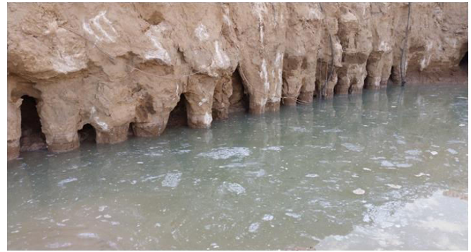
Fig. 8 Subsurface Water Filling the Site and Erode the Sand Layer Creating Cavities behind the Shoring Piles.
